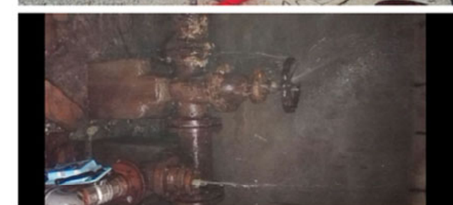
Leak (in a well) on Via Gregorio XI
